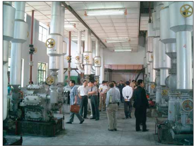
A visit to the engine room at the Wujing Cold Storage Company was part of a tour conducted as part of a WFLO seminar in Shanghai, China.
